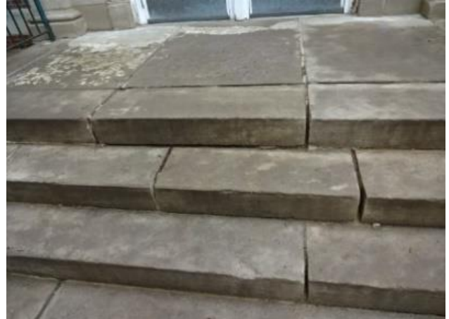
East Steps to be Repaired
