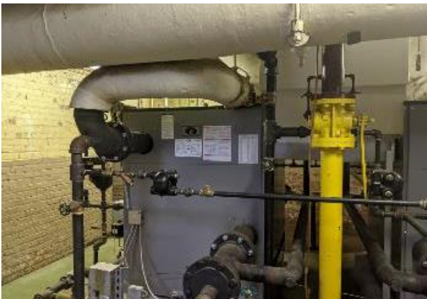
Steam Boiler Serving Entire Building
