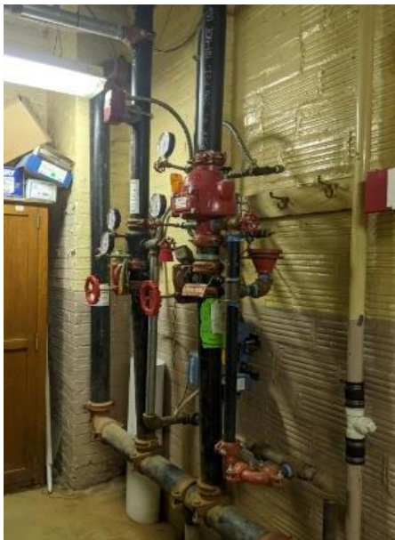
Fire Suppression Equipment in Original Building
