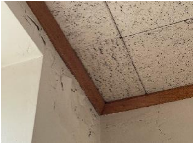
Wall and Ceiling Condition
