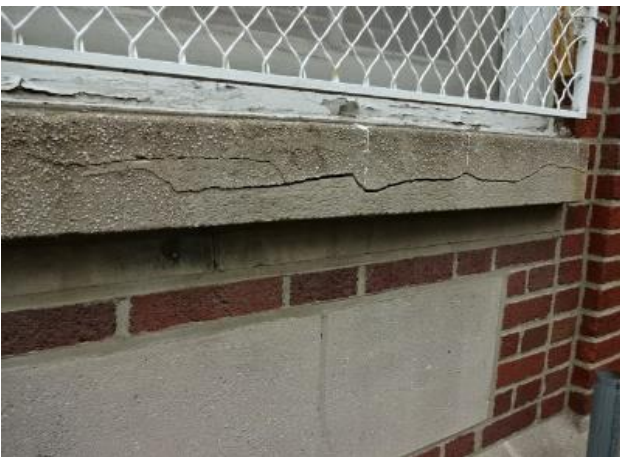
Crack to be Repaired
