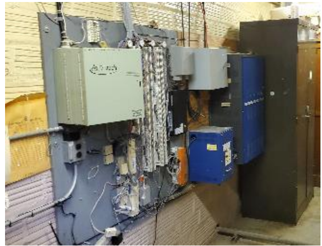
Main Telecom Service
