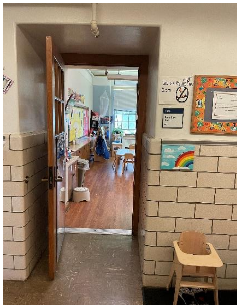
Non-ADA Compliant Clearances
