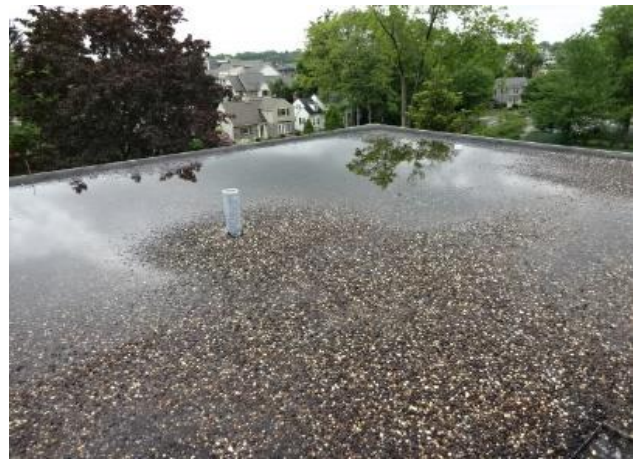
Roofing to be Replaced
