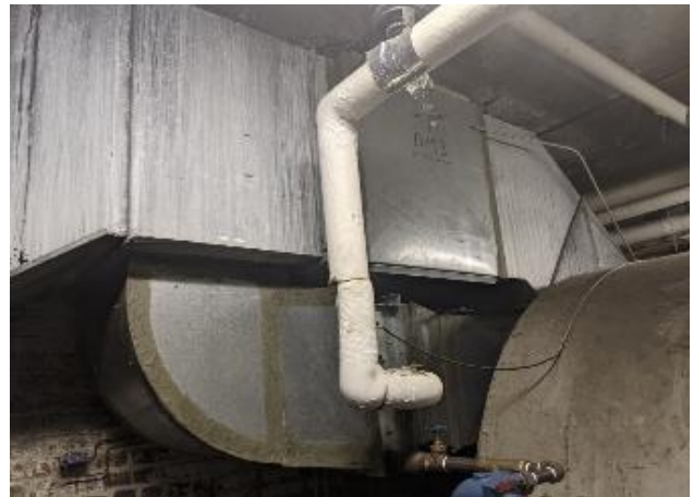
Gym Ventilation Ductwork with Bypass and Coil
