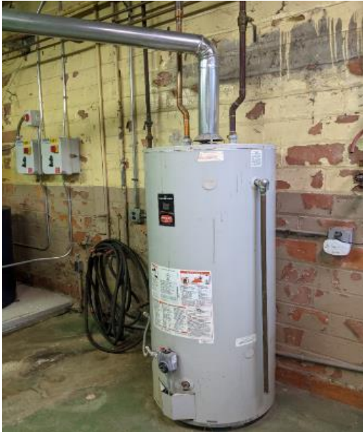
Hot Water Heater in Original Building
