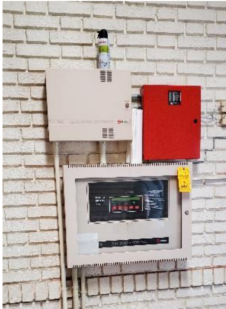
Main Fire Alarm Panel
