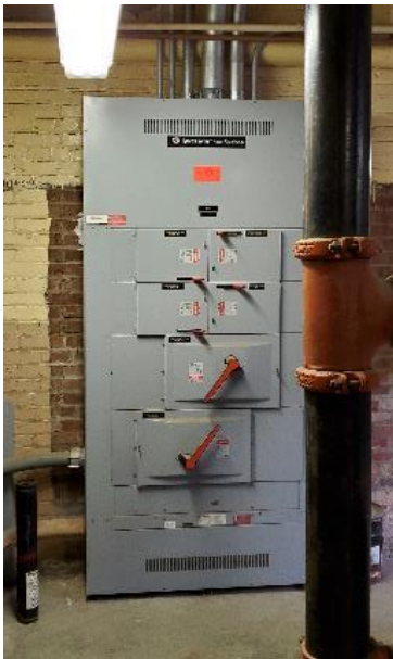
Main Electrical Panel
