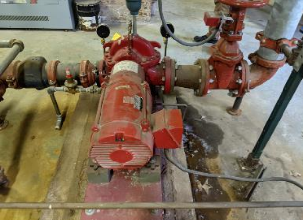
Fire Suppression Equipment in Addition
