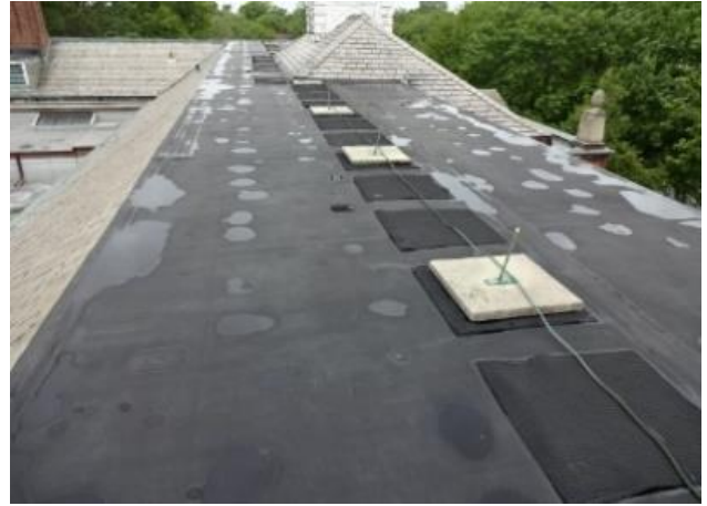
Roofing to be Replaced
