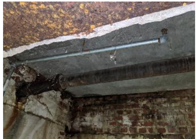
Sanitary Pipe in Coal Storage Room
