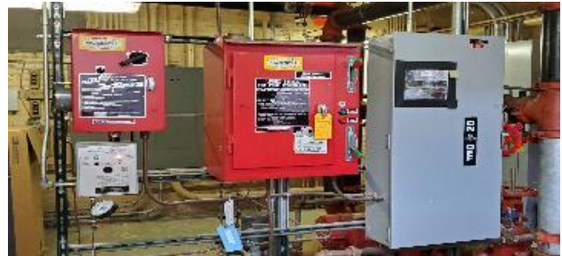
Fire Pump Electrical Equipment
