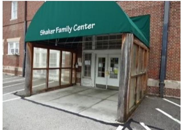
Canopy Structure to be Repaired
