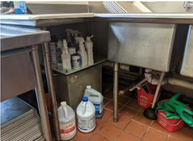
Kitchen 3-Compartment Sink with Grease Interceptor
