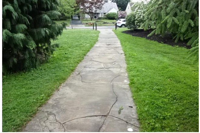
Sidewalk to be Replaced
