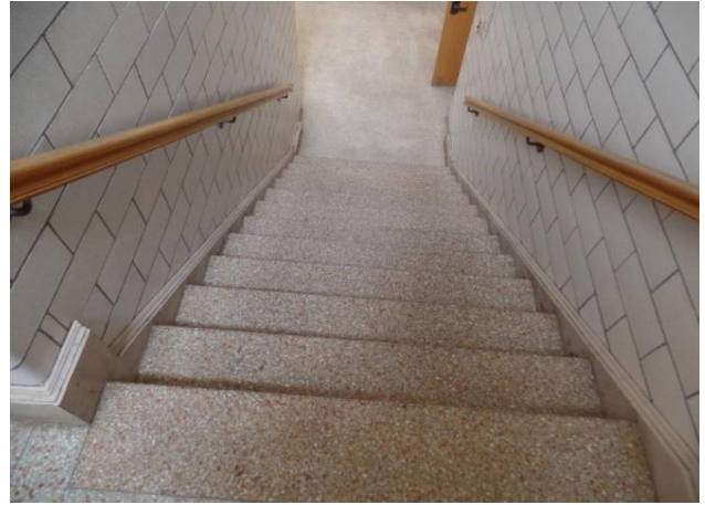
Handrails to be Replaced
