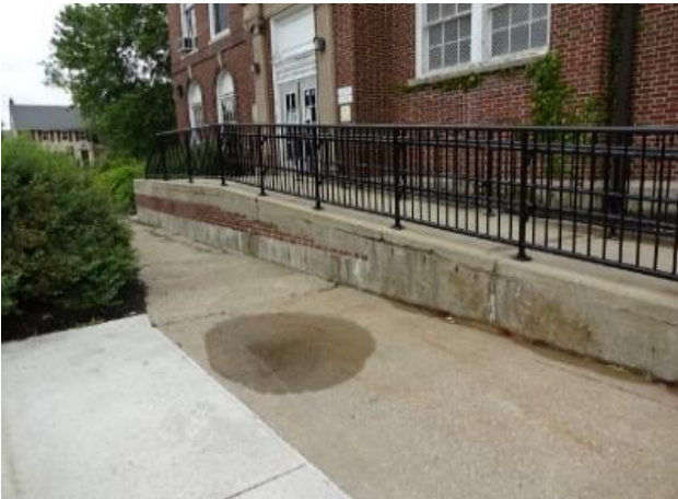
East ADA Ramp to be Repaired
