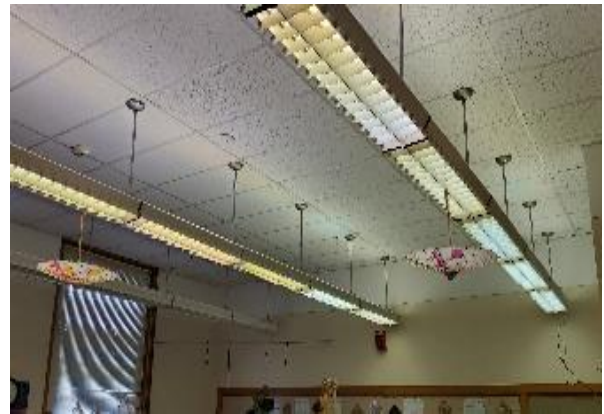
Typical Classroom Lighting
