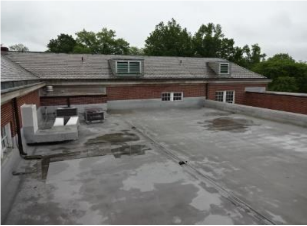
Roofing to be Replaced
