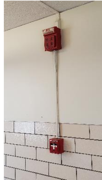
Pullstation and Notification Device
