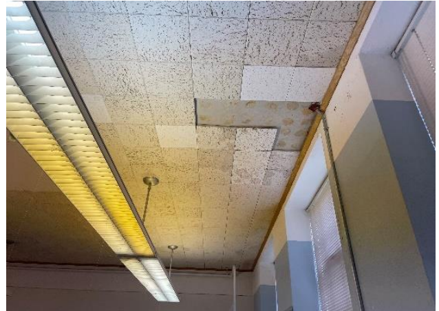
Missing Ceiling Tiles
