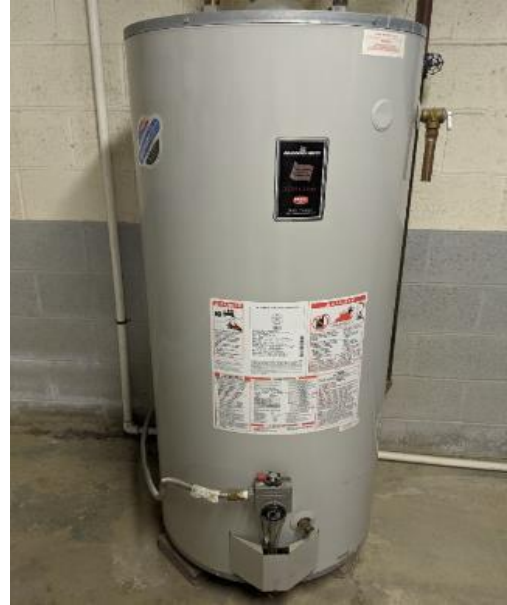
Hot Water Heater in Addition Mechanical Room
