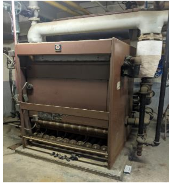
Boiler in Addition Mechanical Room
