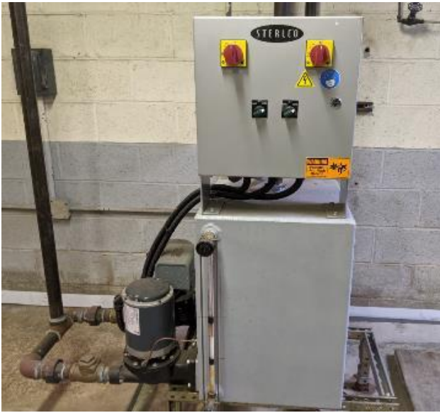
Steam Condensate Pump in Addition Mechanical Room
