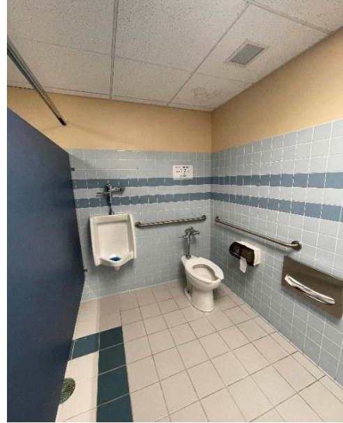
Basement Level Restroom with Extra Fixture
