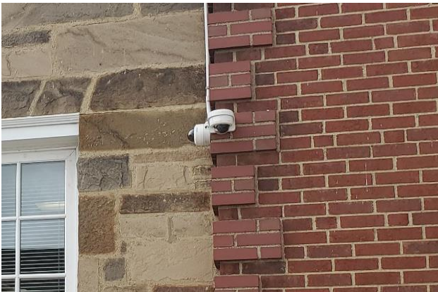
Exterior Security Cameras
