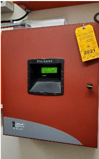
Main Fire Alarm Panel
