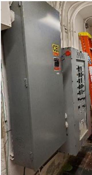
Main Electrical Disconnect
