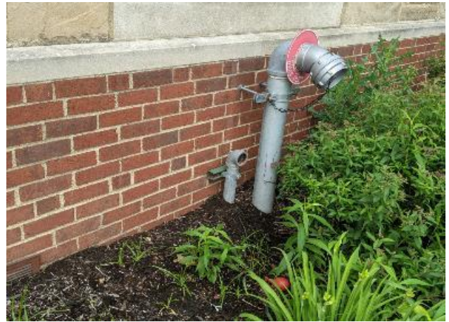
FDC on Side of Building
