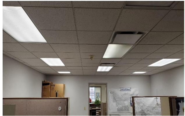
Typical Office Lighting
