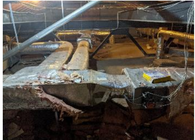
Terminal Unit and Missing Insulation
