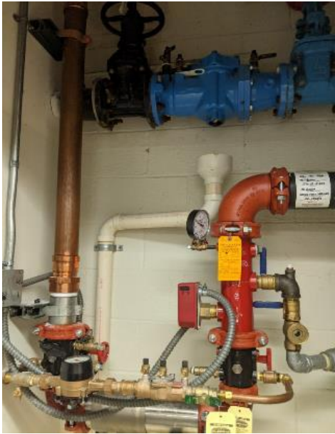
Fire Suppression System
