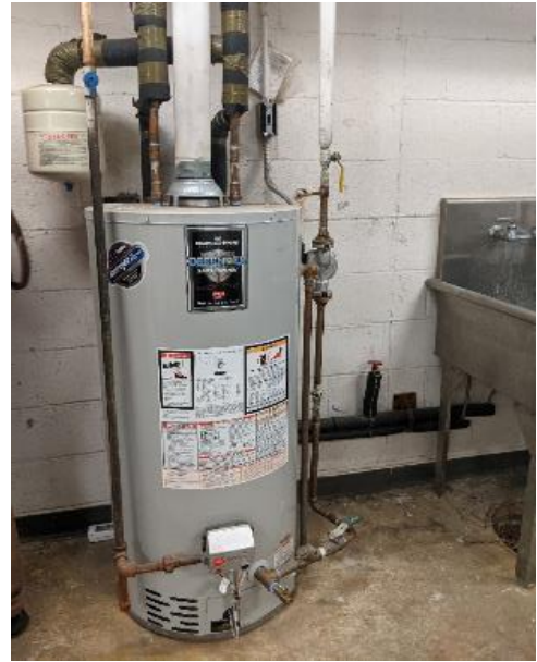
Building Water Heater
