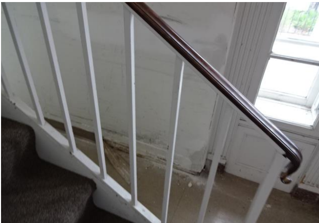
Handrail to be Replaced
