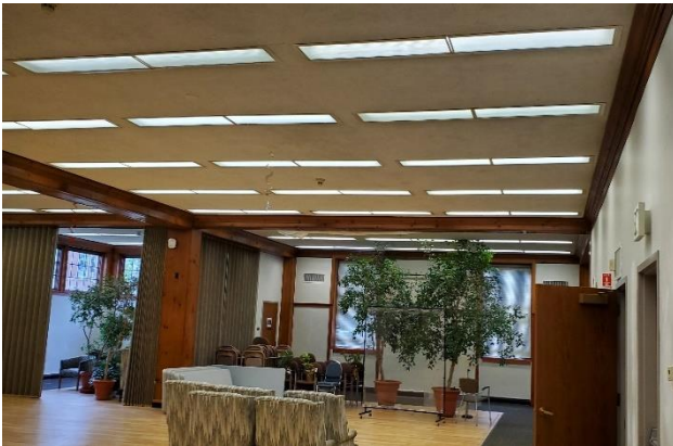
1st Floor Assembly Lighting
