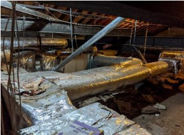
Furnace and Dented Ductwork
