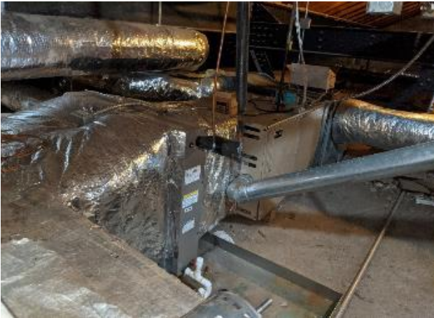
Gas Fired Furnace in Attic
