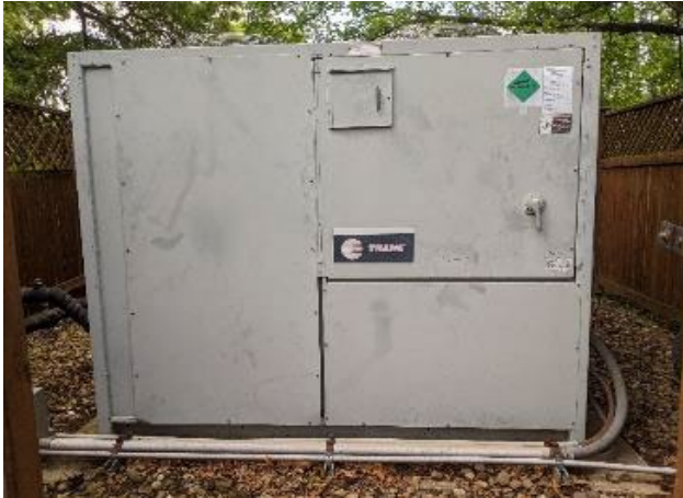
Outdoor Air-Cooled Chiller
