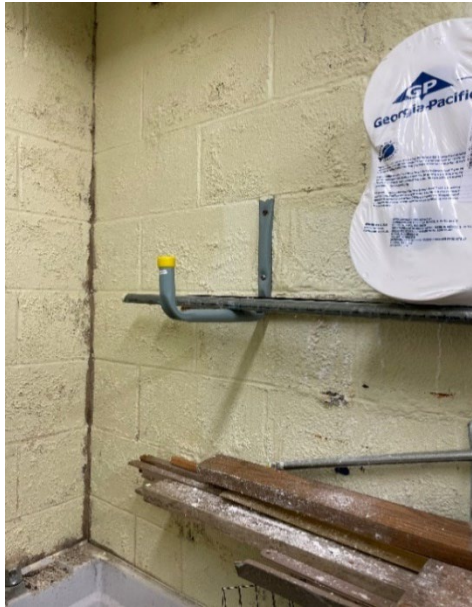
Peeling Paint at Foundation Wall
