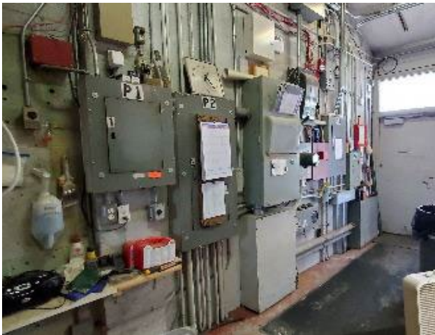
Main Electrical Equipment
