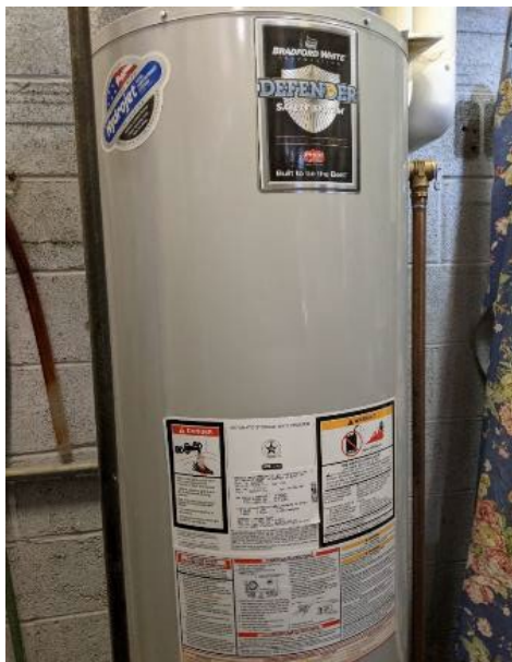
Hot Water Tank
