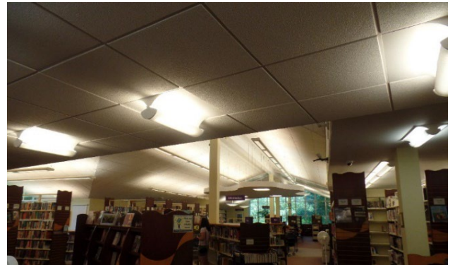
Surface T8 Fixtures
