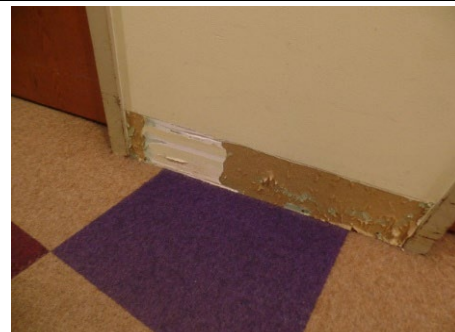
Corridor Wall Base Condition
