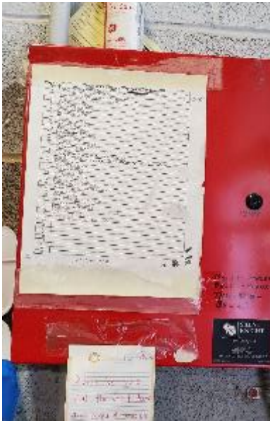
Main Fire Alarm Panel
