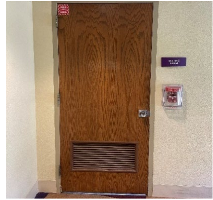
Non-Compliant Knob Hardware
